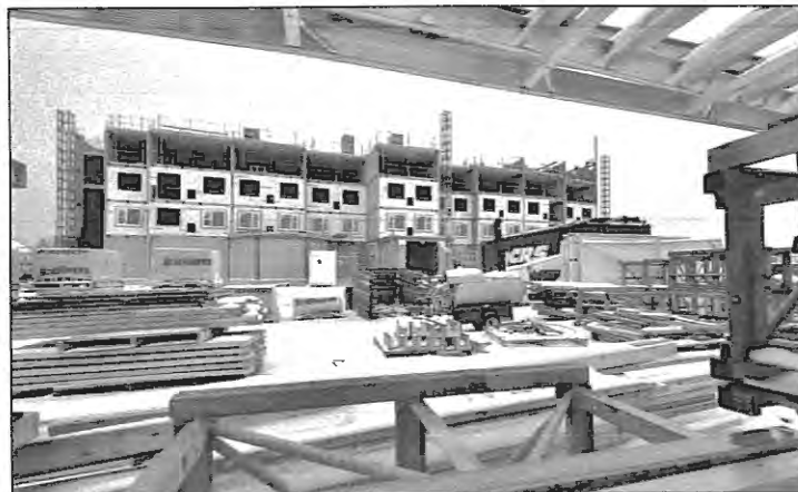
Three rental projects, including this one in Collingwood, will create an additional 257 units of affordable housing in the County (2019-2020).
