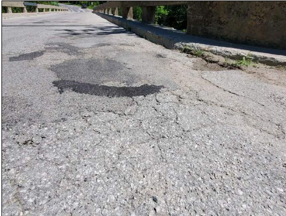
Patches and map cracking on approach wearing surface (typ.)
