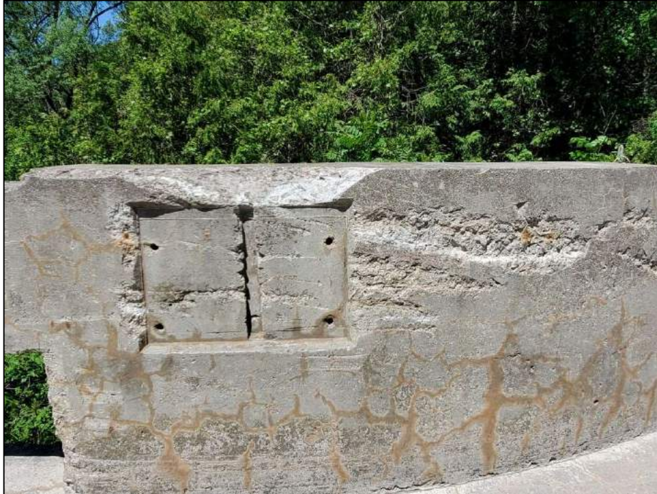
Scaling on North-West barrier end post.
