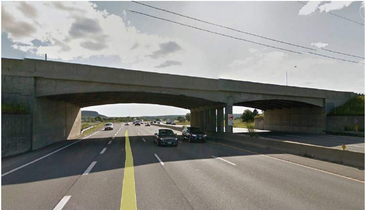
Figure 8: Esquesing Township Bridge No. 5, a two-span T-beam structure built in 1960 (Google Streetview)
