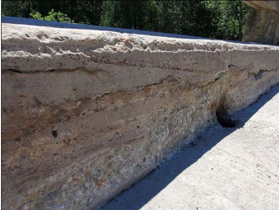
Medium crack and abrasion damage along interior face of North curb.
