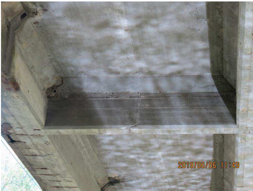
IMG_1692 Cracks in Diaphragm
