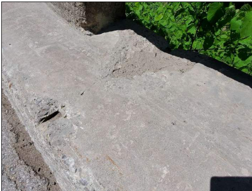
Spall on top face of East curb.
