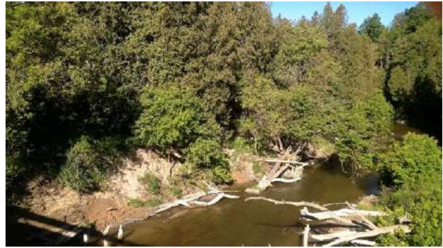
Photo 2. Facing approximately southwest downstream of bridge; note eroded sections of south bank adjacent to bridge (June 17, 2021).
