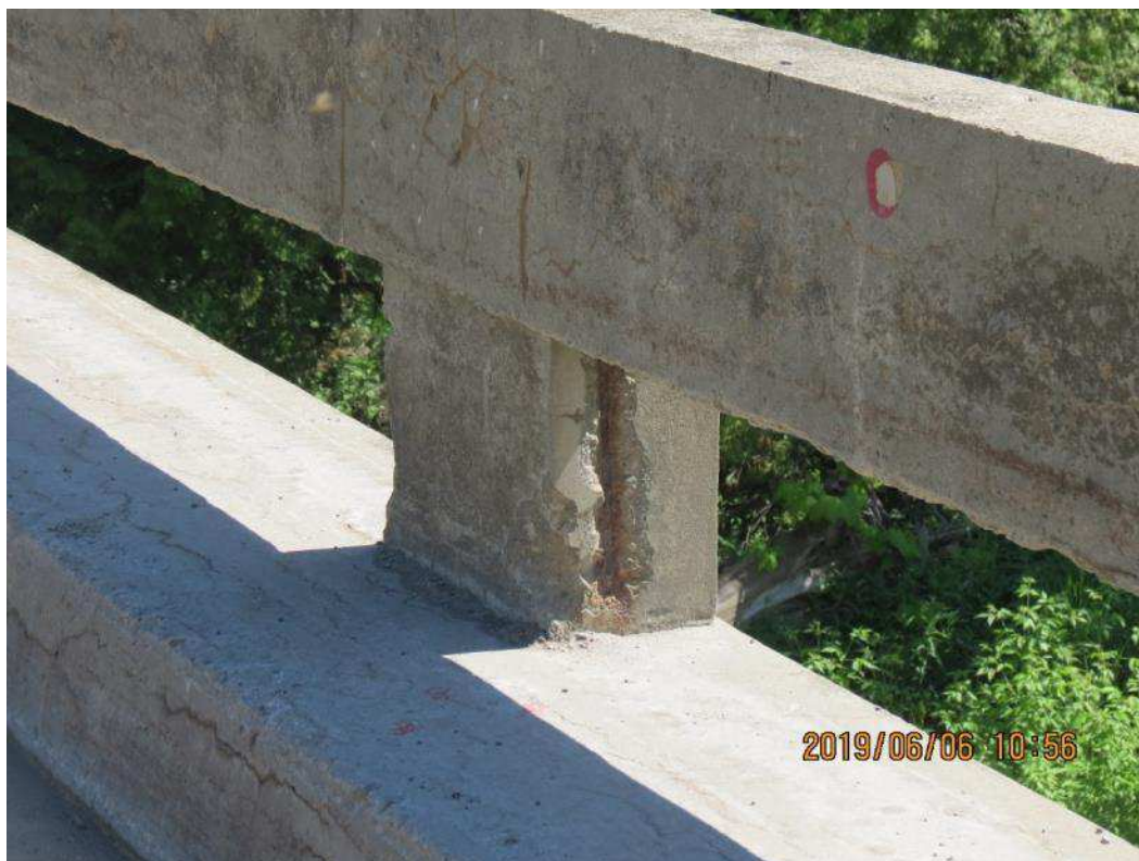
IMG_1495 Post with Exposed Rebar
