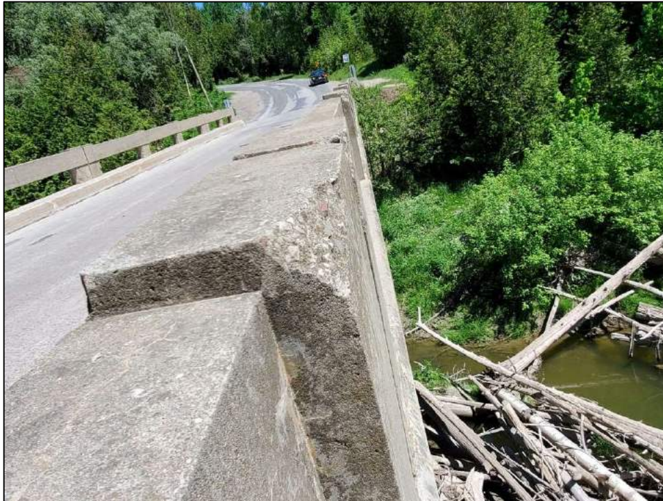
Spall at top corner of intermediate barrier post (typ.)
