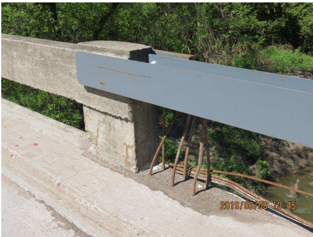
IMG_1403 Missing Concrete Post
