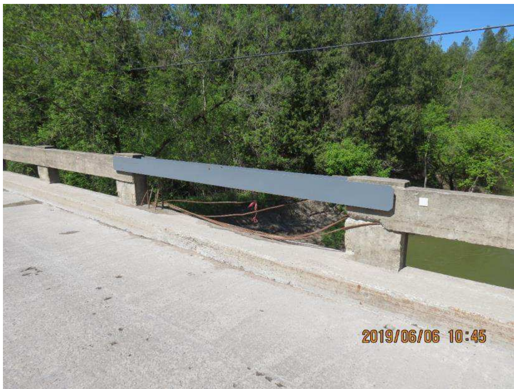
IMG_1401 West Railing Missing Section
