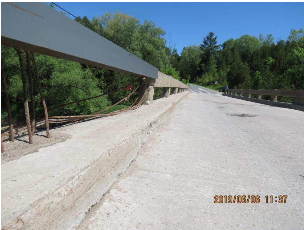
IMG_1628 West Curb at Missing Railing
