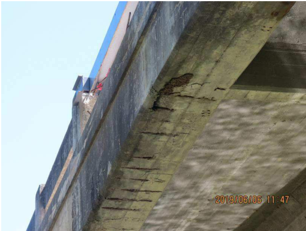
IMG_1674 Typical Exposed Rebar and Deterioration of Girders
