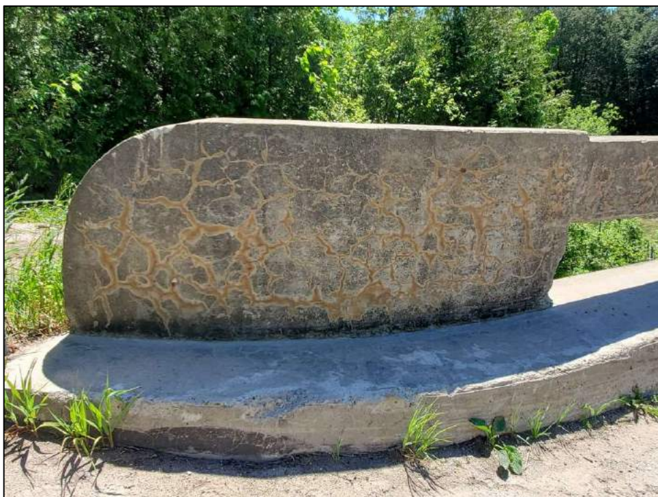
Map cracking on barrier end posts (typ.)
