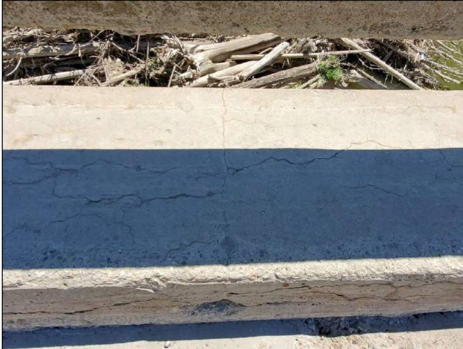
Map cracking top face of curb (typ.)
