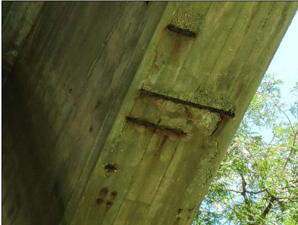
Delamination and spall with exposed rebar at bottom of exterior T-beam (typ.)
