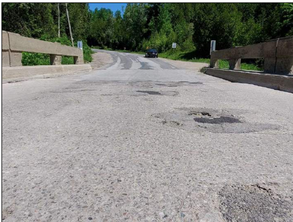
Asphalt patches on deck wearing surface (typ.)
