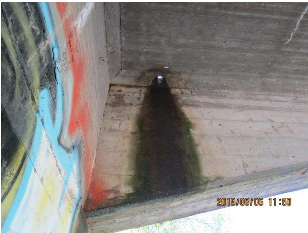
IMG_1701 Typical Deck Drain Surface Deposit
