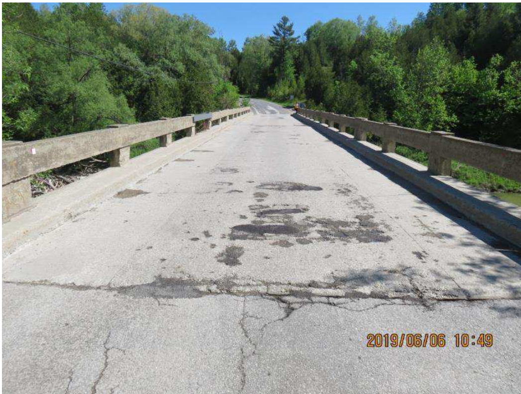
IMG_1434 South Deck Joint (1 of 2)
