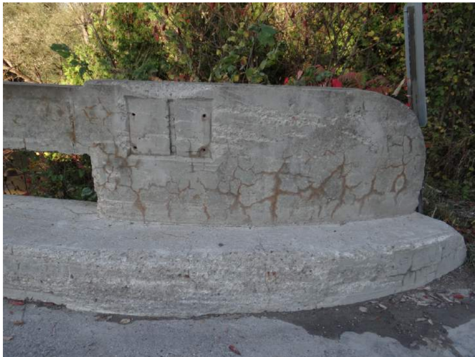
Plate 13: West railing on north approach, showing where the plaque for the bridge was originally located, looking west.
