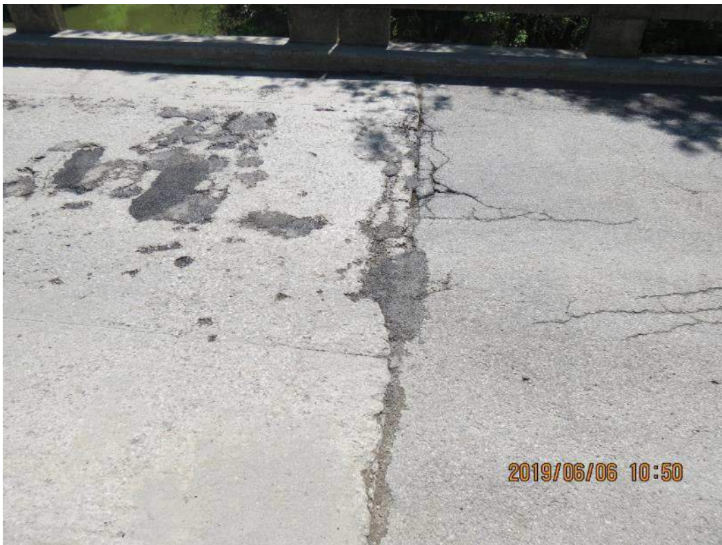
IMG_1437 South Deck Joint (2 of 2)
