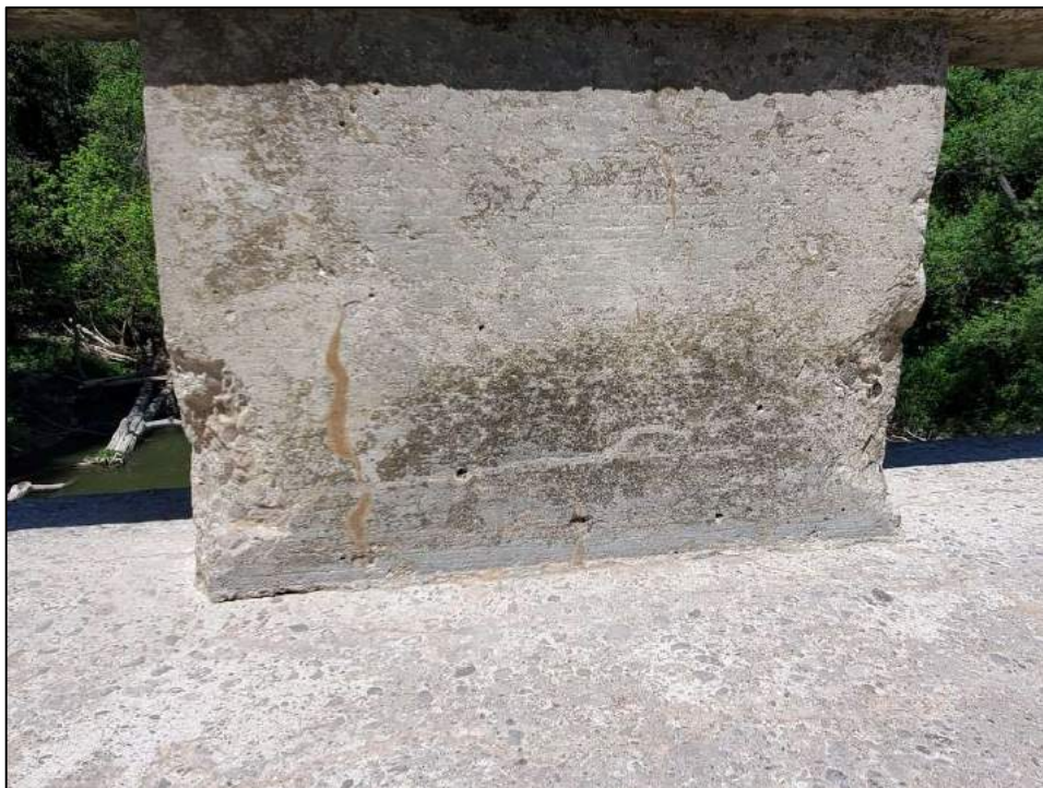
Spalls at bottom corners of intermediate barrier post (typ.)
