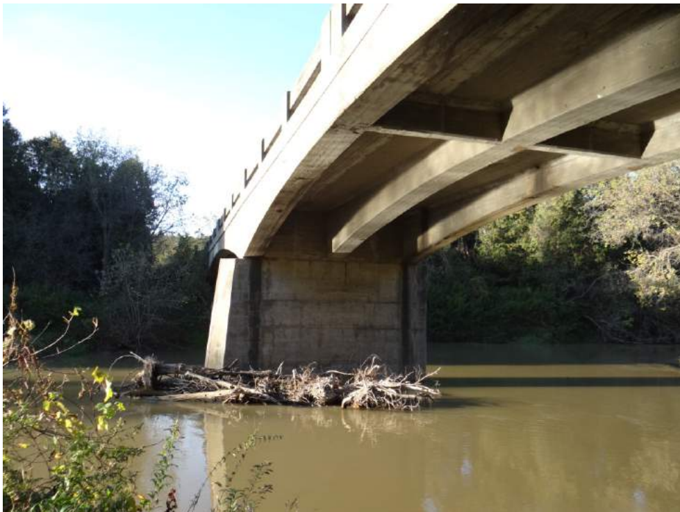
Plate 6: East elevation showing soffit and north elevation of central pier, looking southwest.
