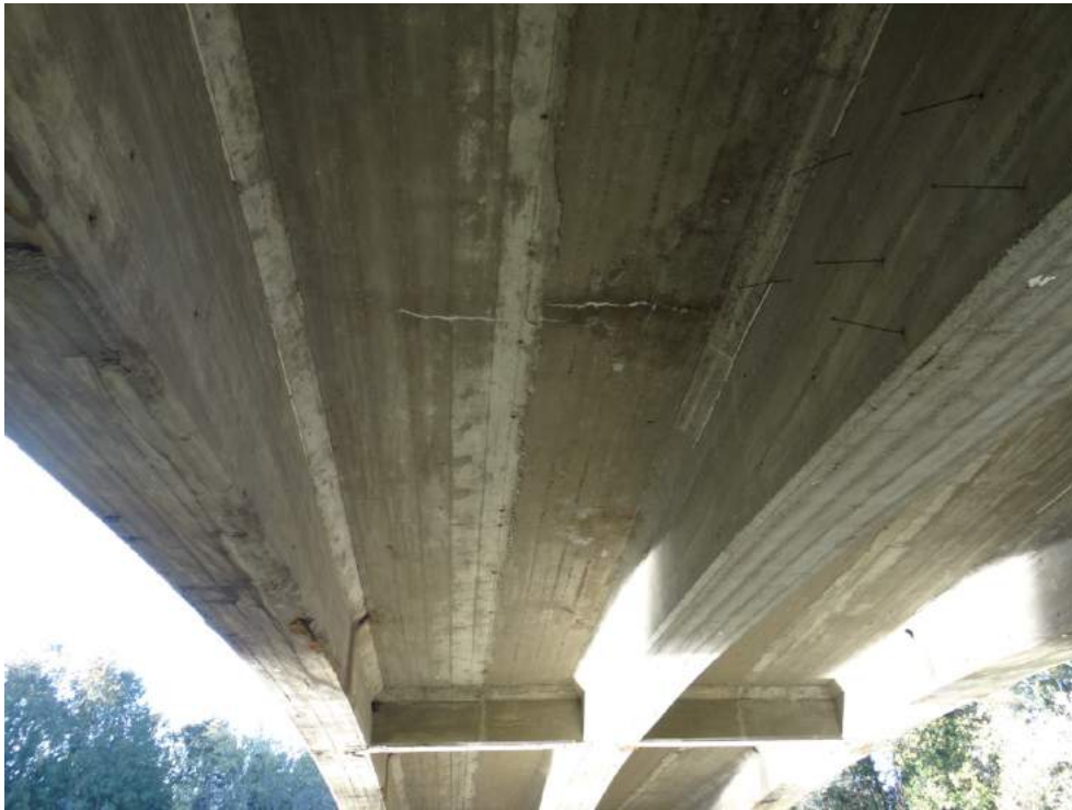
Plate 7: Bridge soffit showing variable-depth arched T-beams and cast-in-place concrete deck, looking south from north abutment.
