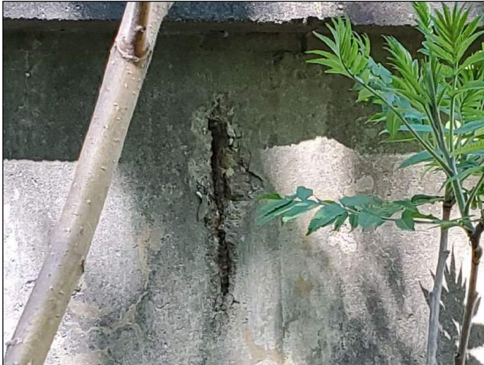
Delamination and spall with exposed rebar South-East wing wall.
