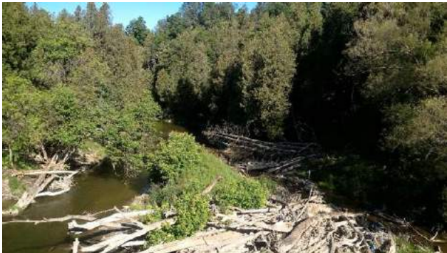
Photo 3. Facing west downstream of bridge; downstream extent of large log-jam surrounding bridge (June 17, 2021).
