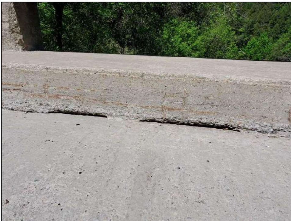
Scouring along bottom of curb.
