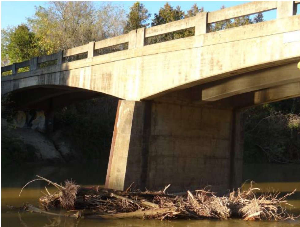
Plate 5: East and north elevations of the central pier, looking southwest. Note the ice floe protection on the upstream side of the pier.
