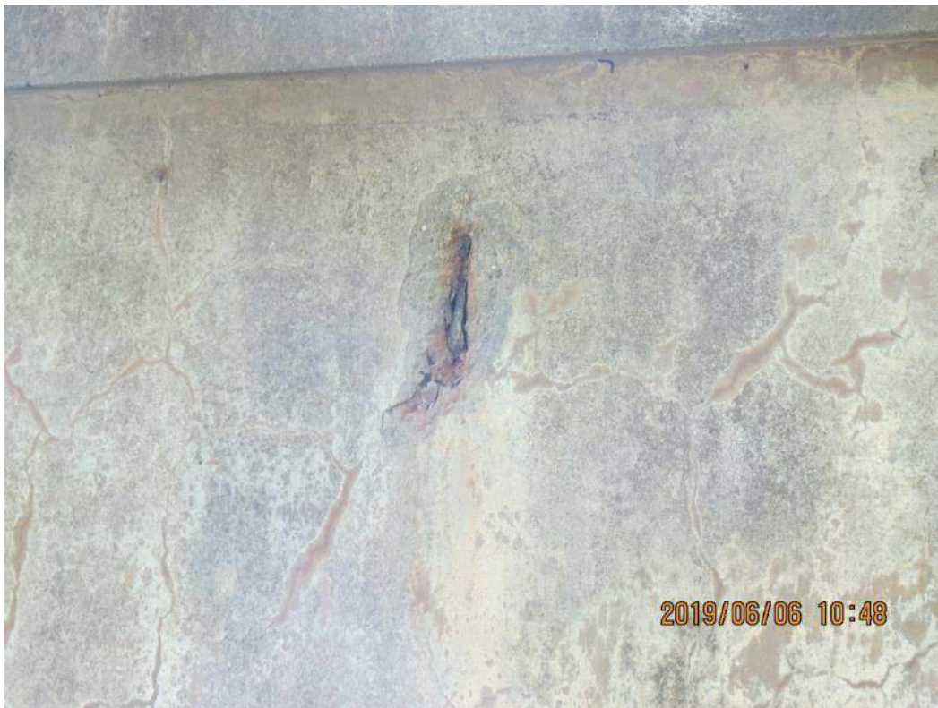
IMG_1424 Typical Wingwall Exposed Rebar
