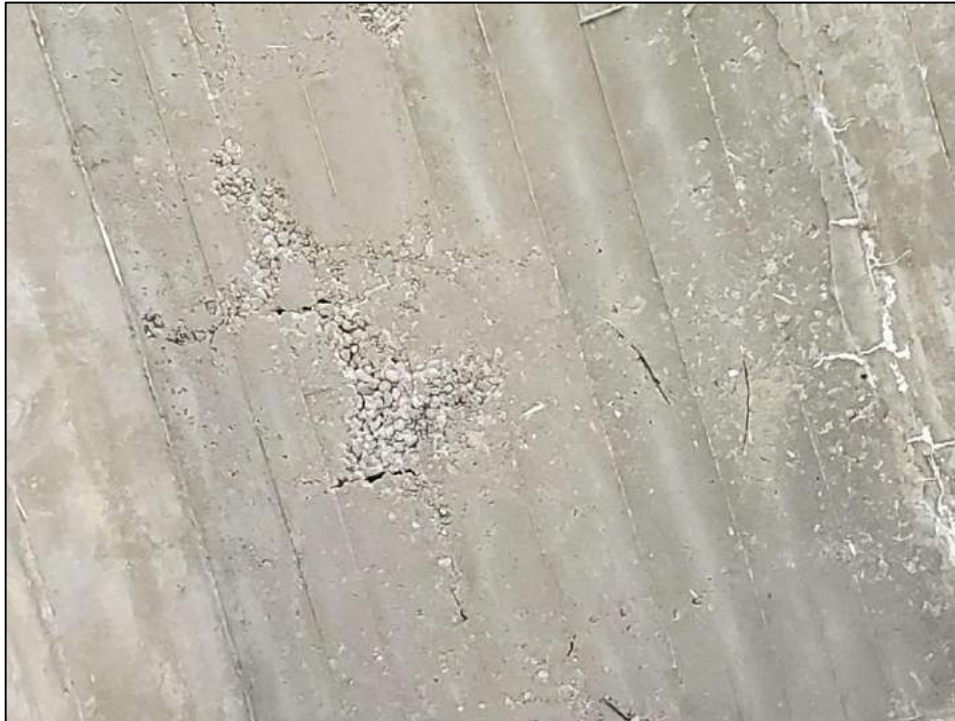
Localized honeycombing interior soffit.
