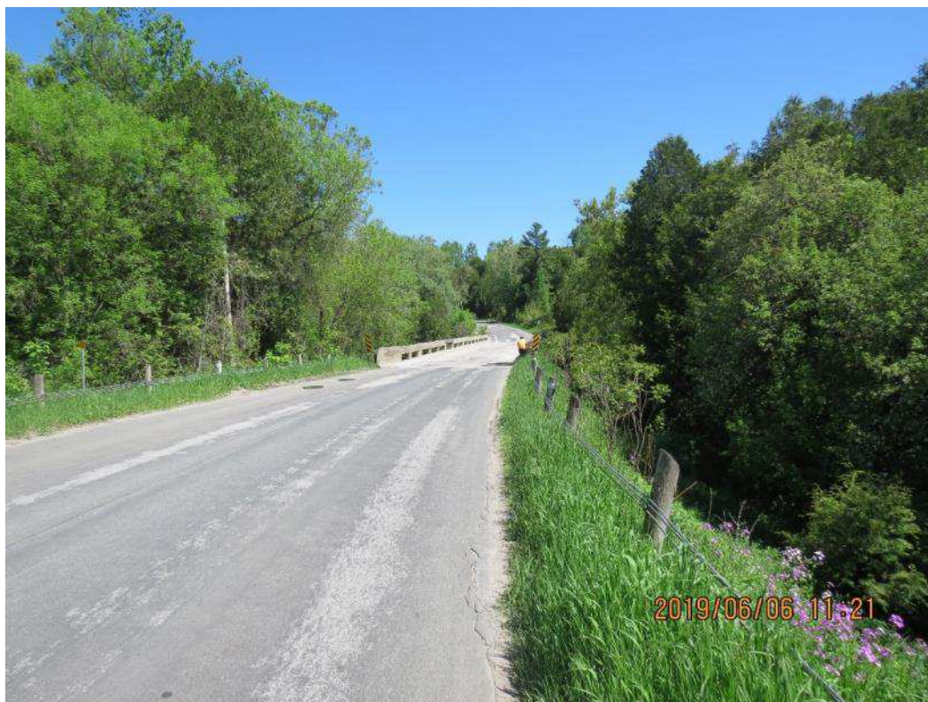
IMG_1607 Typical Southeast Cable Guide Rail
