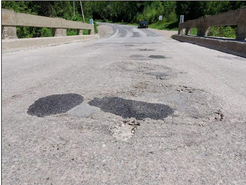
Potholes on deck wearing surface (typ.)
