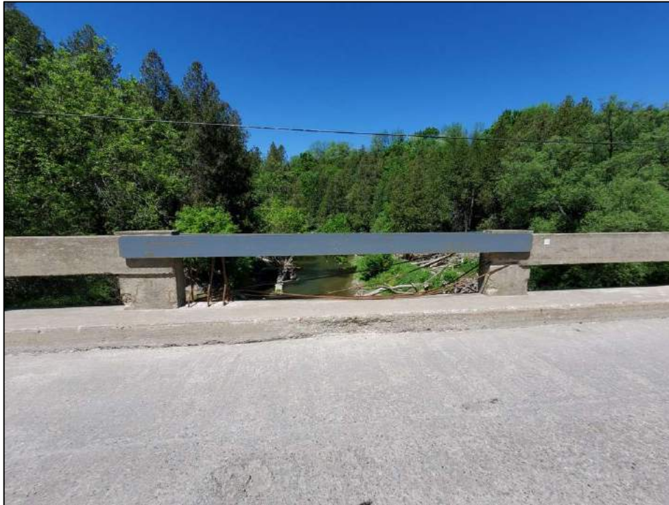
Missing section at midspan of West railing replaced by I-Beam.
