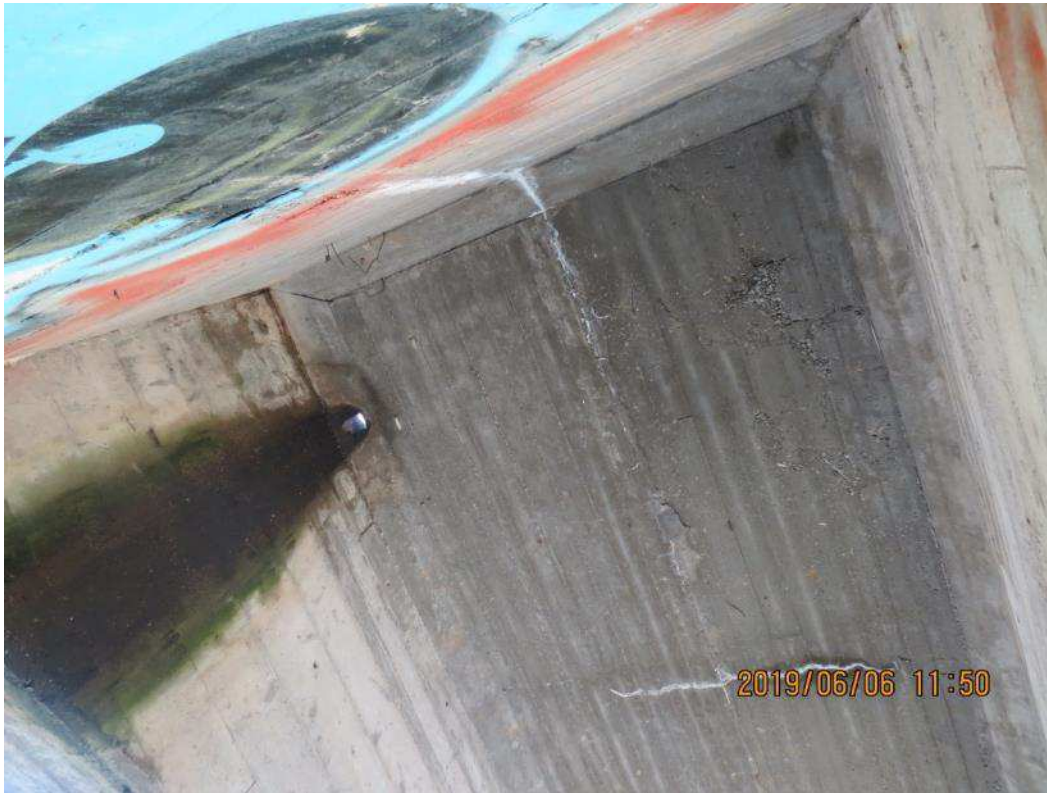
IMG_1700 Typical Soffit Deficiencies (1 of 2)
