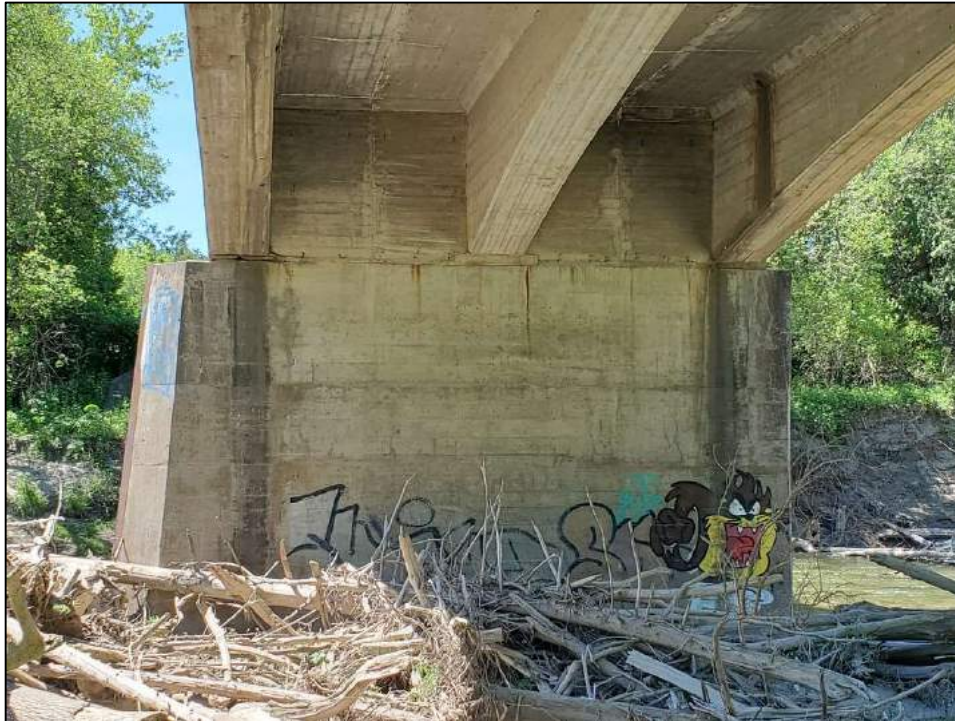
Medium crack with efflorescence at centre of pier diaphragm (typ.)
