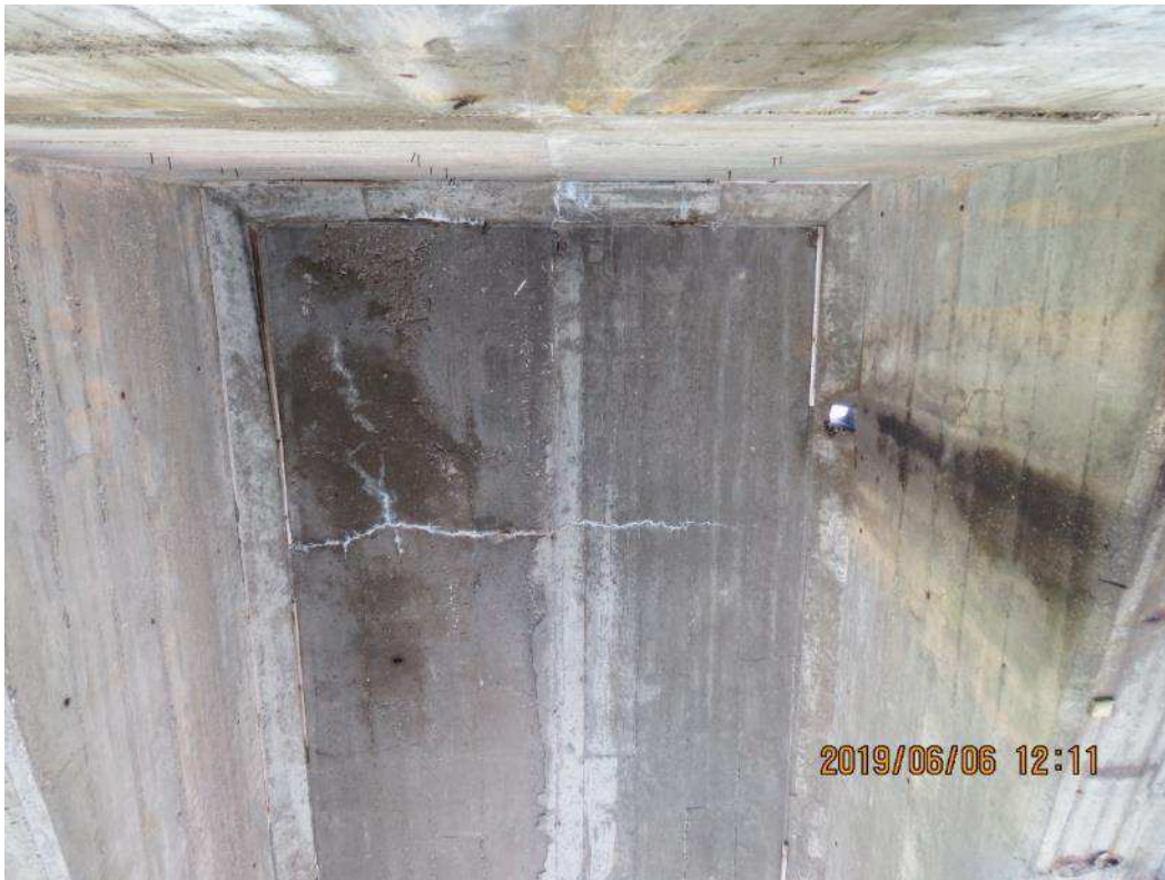
IMG_1797 Typical Soffit Deficiencies (2 of 2)
