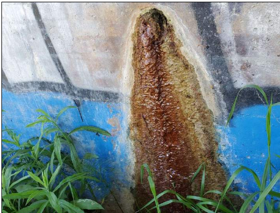
Localized rust stain (typ. of North abutment)
