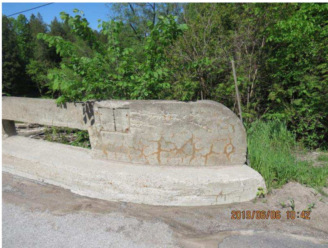
IMG_1378 West Railing North End Panel
