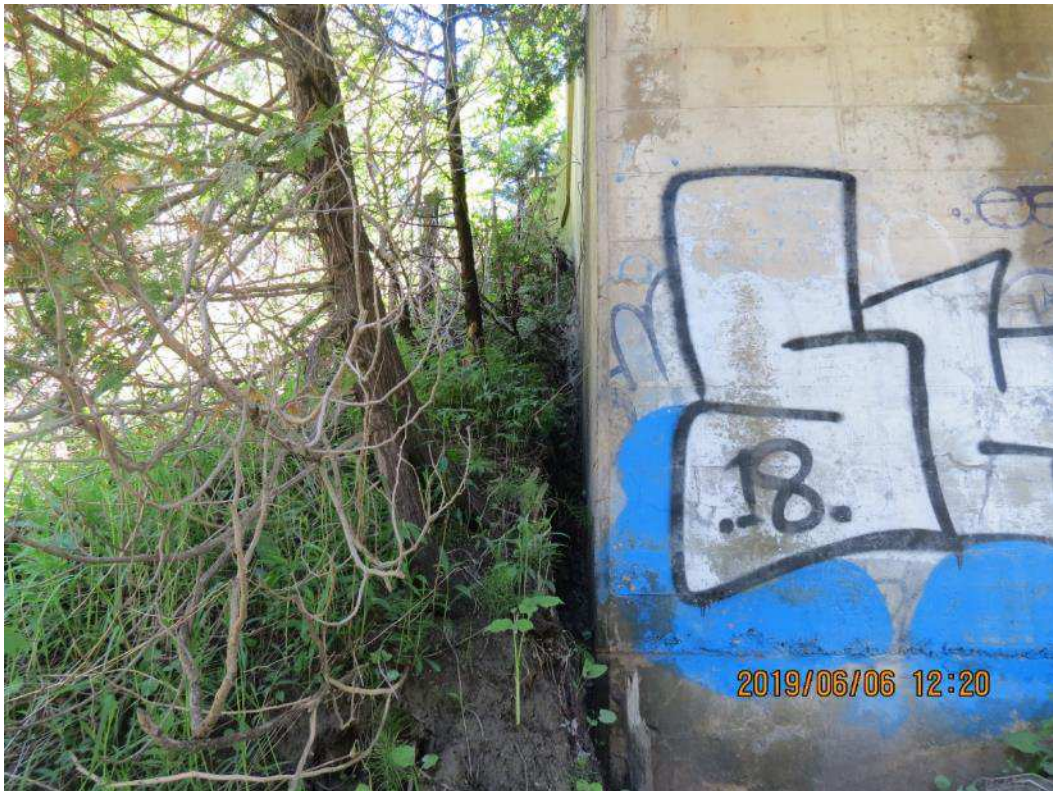
IMG_1851 Northwest Wingwall Minor Washout
