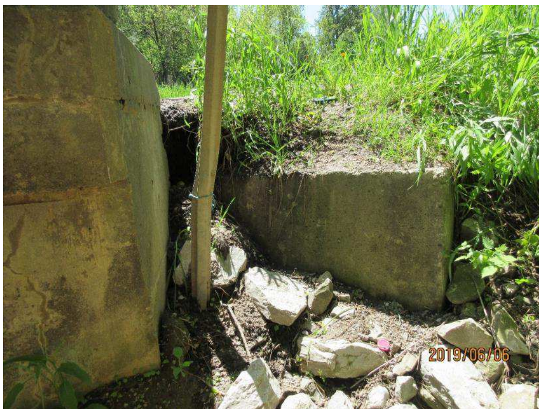
IMG_4709 Exposed Guy Cable Anchorage
