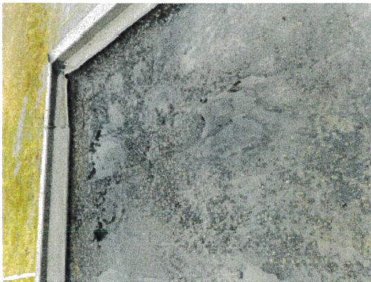
Failed roof membrane
