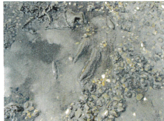
Failed roof felts
