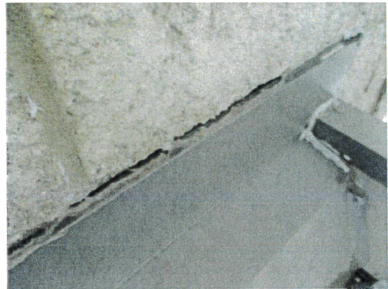
Failing metal flashings
