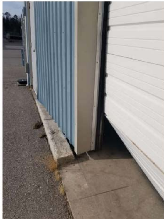
Photograph 2 - Wood Stud Wall Detached from Foundation
