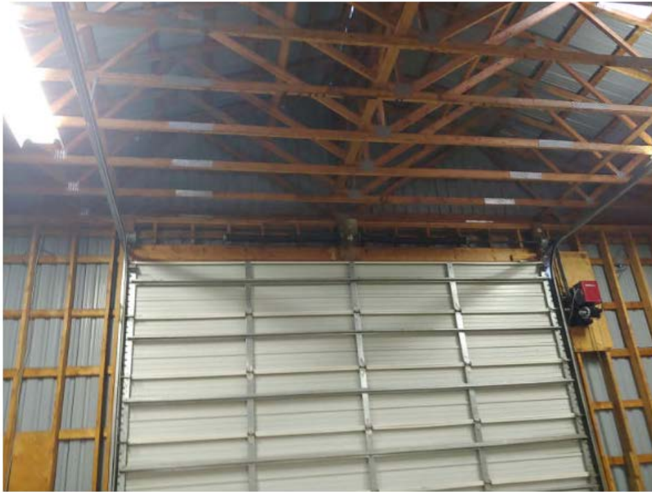
Photograph 7 - Inadequate king studs at each side of the garage door
