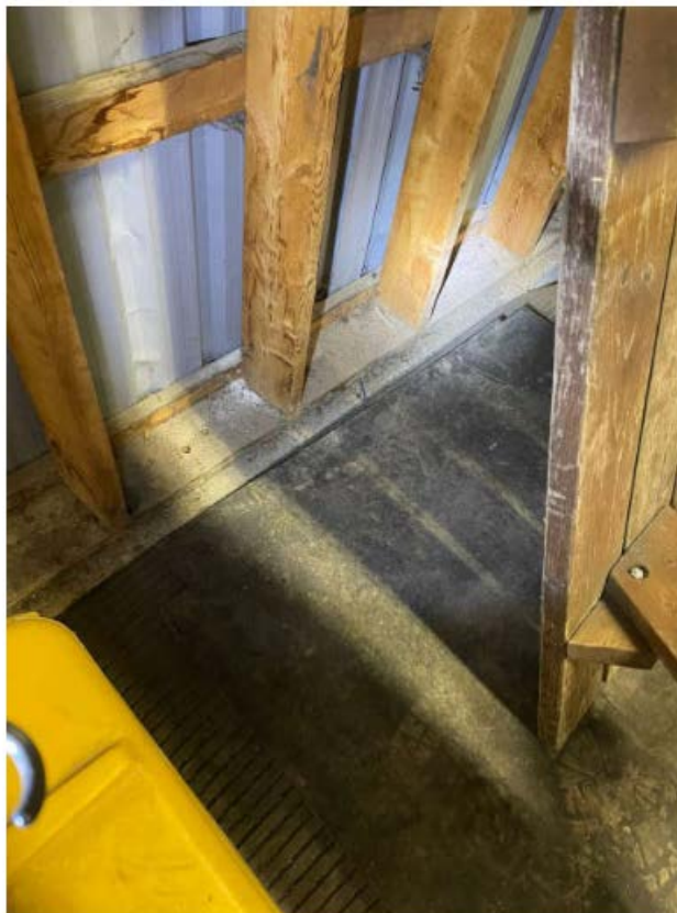
Photograph 8 - Missing sill plate anchorage
