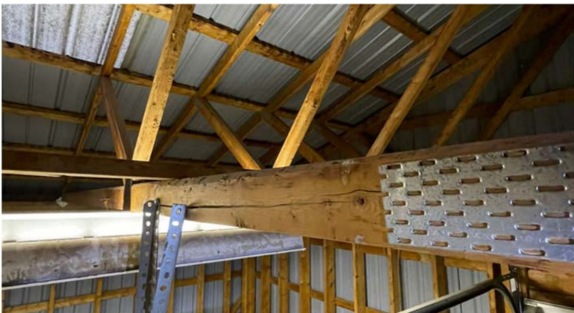
Photograph 4 - Damaged truss bottom chord at 5 th truss from south end
