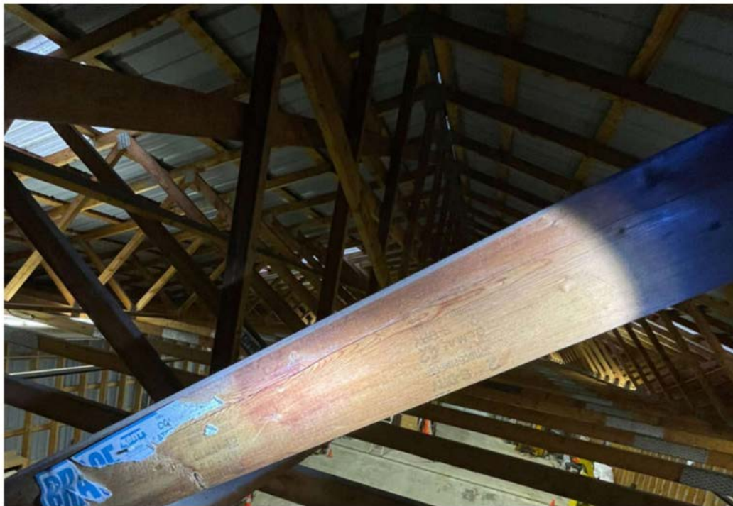
Photograph 6 - Example of narrow checking
