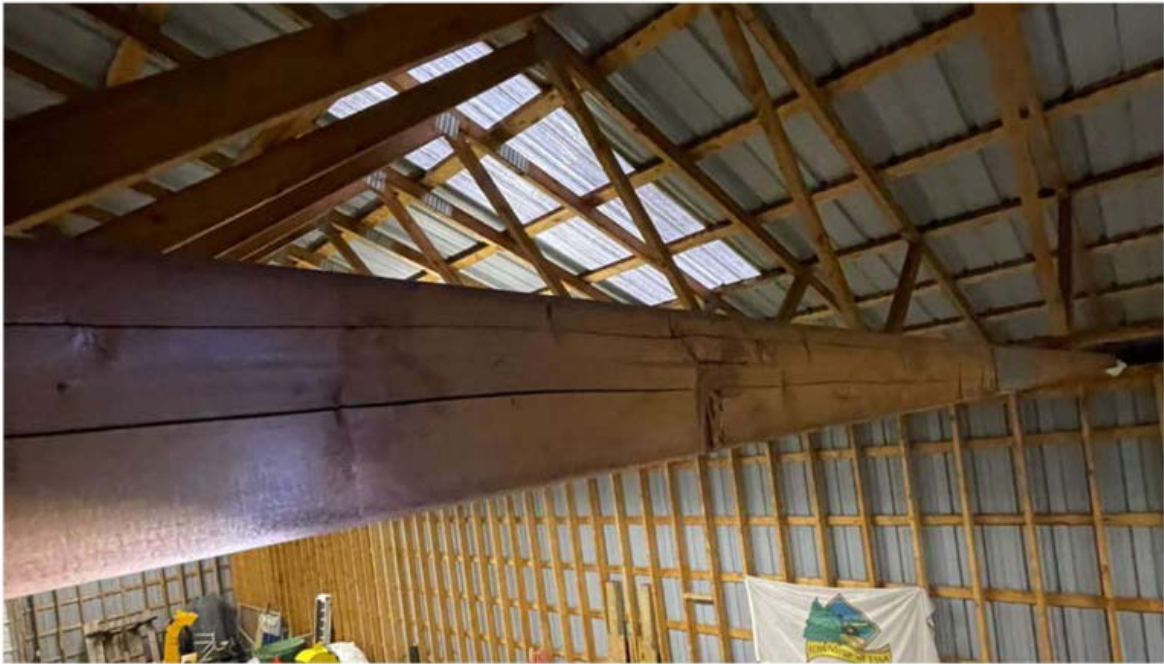
Photograph 5 - Damaged truss bottom chord at 10 th truss from south end
